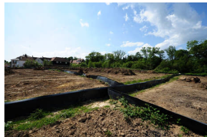
Site clearance underway on the school site, with ‘newt fencing’ to stop newts and reptiles returning
